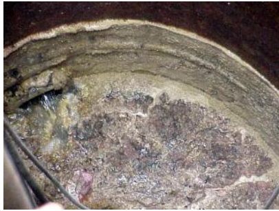
Grease can cause a scum layer to build up on the sidewalls of the lift station.
