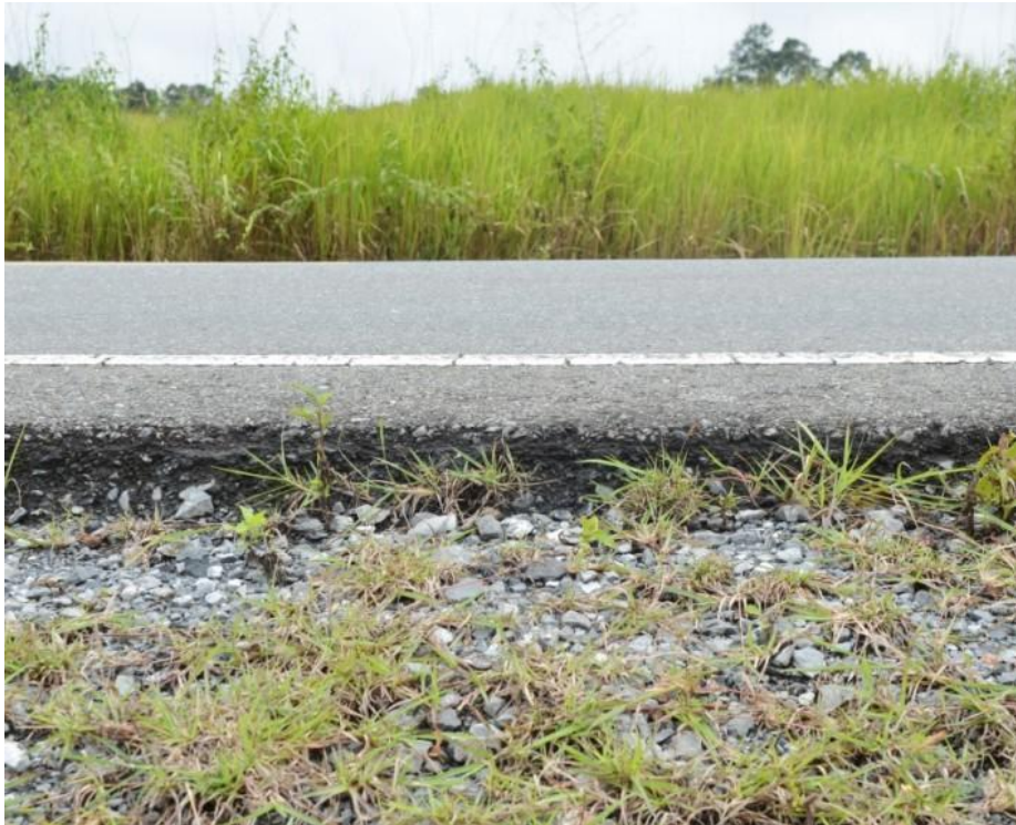
Edge of road drop off
